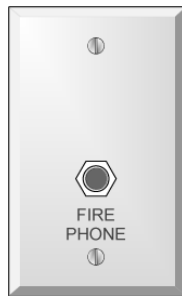
Figure 3: Firefighter Phone Jack Station 976200 Reference
